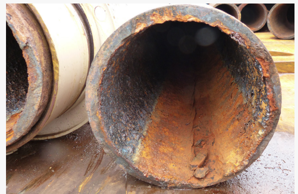
Corroded chrome-iron alloy piping removed from service
