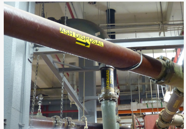
Ash Disposal Header
