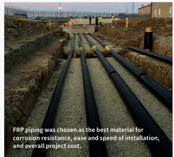
Several thousand feet of Green Thread pipe installed for the correctional facility's cooling water.
